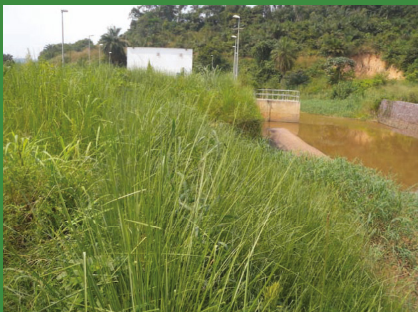
River bank stabilization using vetiver grass. Before (top) and after (bottom) intervention at intake point of the REGIDESO water treatment plant.
