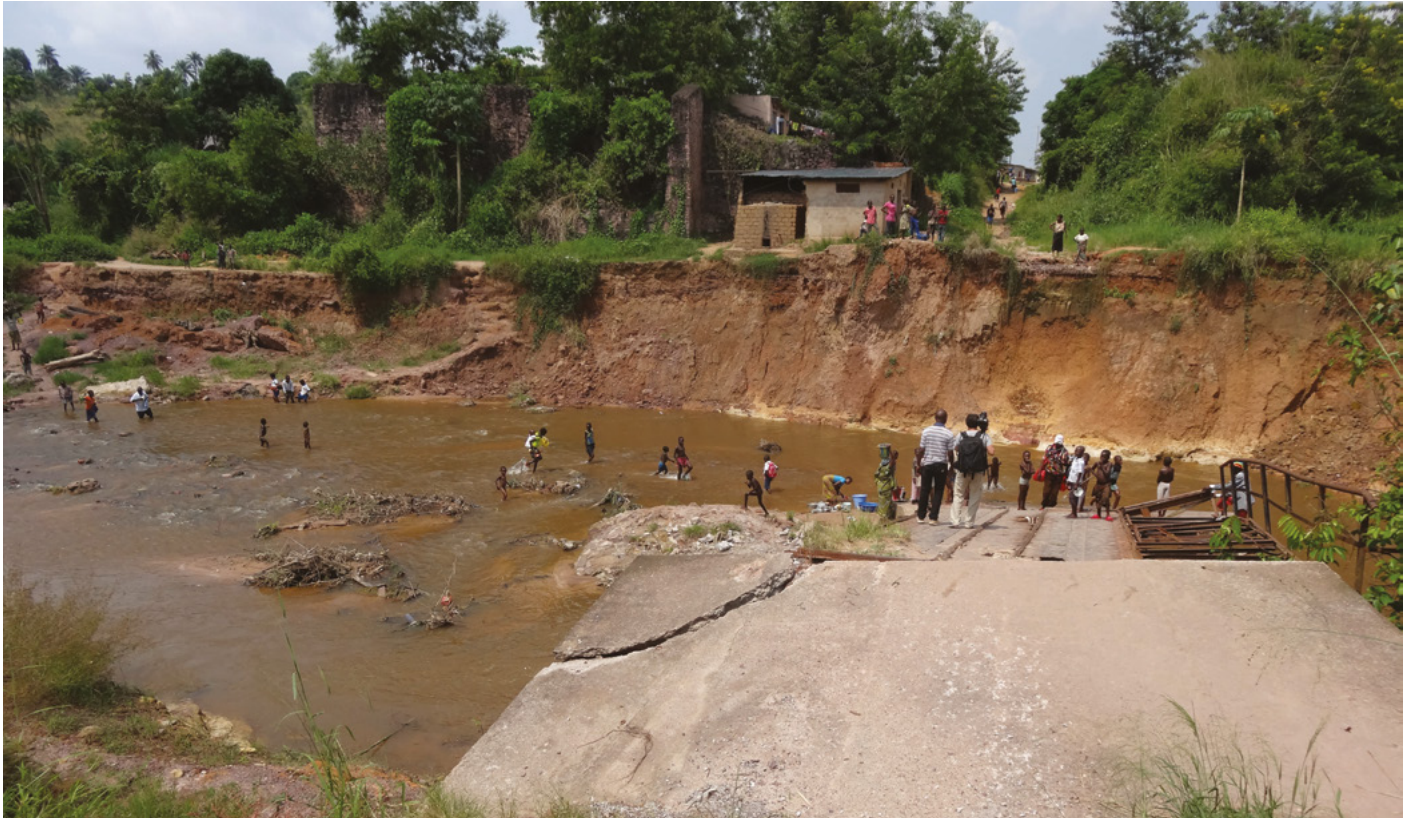
Bridge damaged by 2012 flooding in Kasangulu
