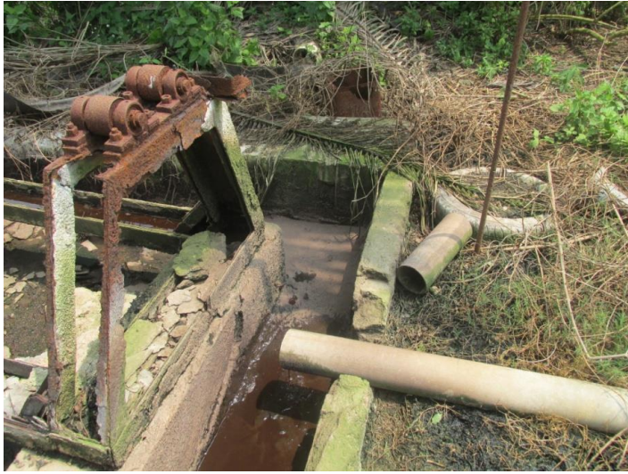
Final Treated Effluent Point
