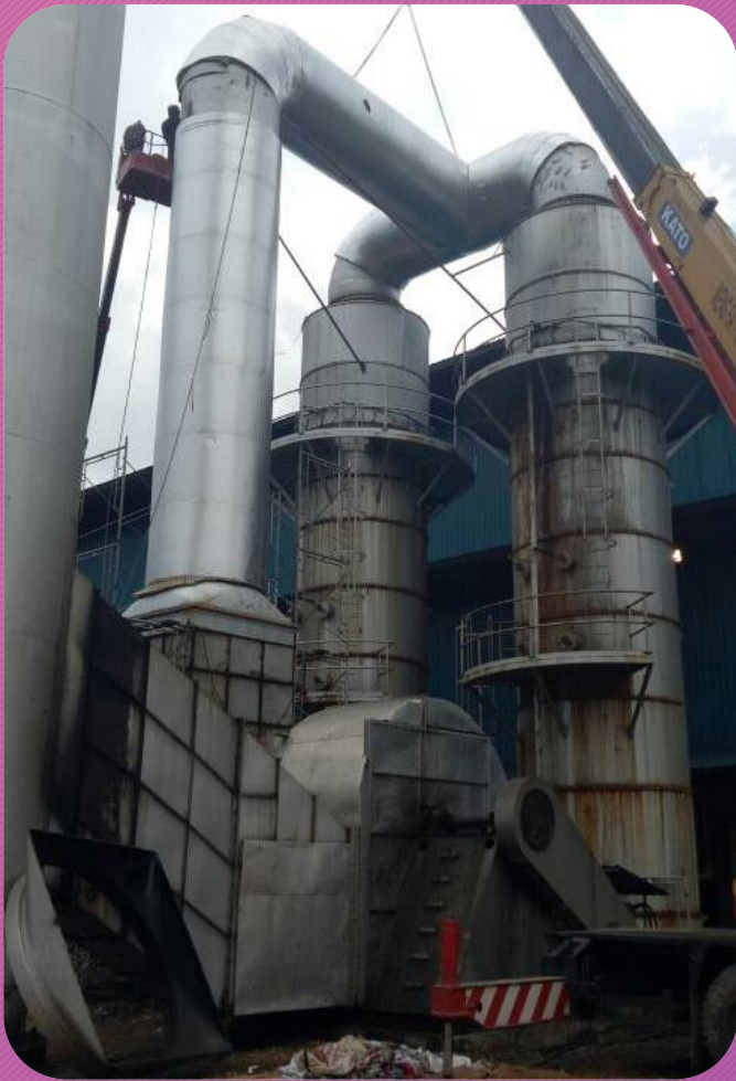
Wet Scrubber Ducting
