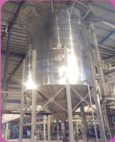
VERTICAL CLARIFIER TANK
