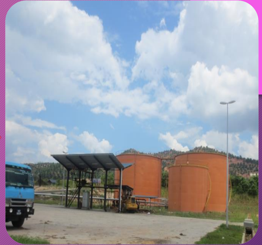
BULK STORAGE TANK (BST)
