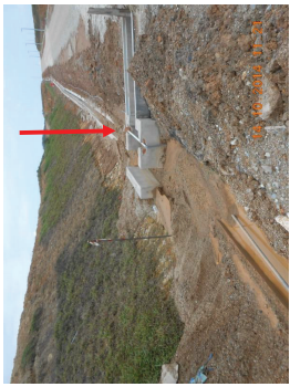
Plate 2a: Silted drain is observed (behind batching plant-access road).
