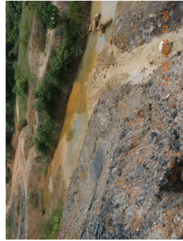
Plate 2b: Silted silt trap has yet to be de-silted (ST-2-06d).
