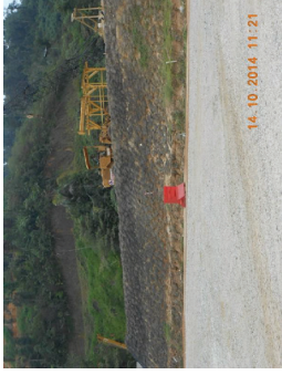
Plate 3c: Turfing has been dead is observed (near to the pipe storage).
