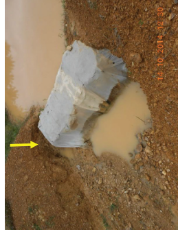
Plate 3b: Gap is observed at gabion wall (ST-2-17).
