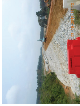
Plate 4b: Exposed slope has yet to be vegetated (relocation road).
