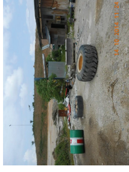
Plate 5c: Poor housekeeping is observed (batching plant).
