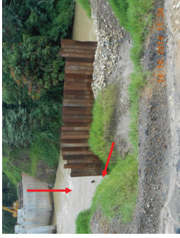
Plate 4a: Eroded embankment of silt trap is observed (ST-2-06e).
