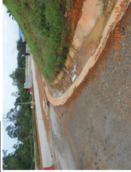
Plate 2a: Silted drain has yet to be de-silted (near main entrance gate).
