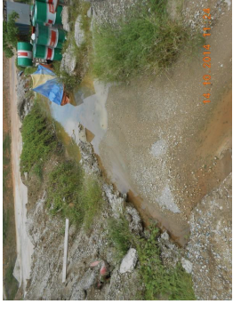
Plate 2b: Silted earth drain has yet to be de-silted (batching plant).
