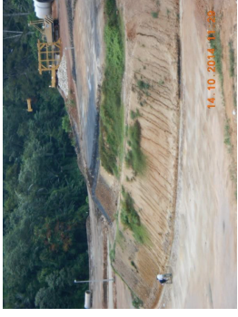
Plate 1d: Exposed slope is observed (Main Dam).
