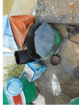
Plate 6a: Poor housekeeping is observed (batching plant).
