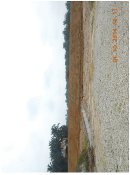
Plate 1i: Exposed slope is observed (LHS CH 2650 relocation road).
