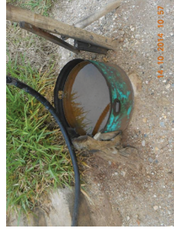
Plate 6c: Contaminated geotextile and oil ponding is observed (workers' camp).
