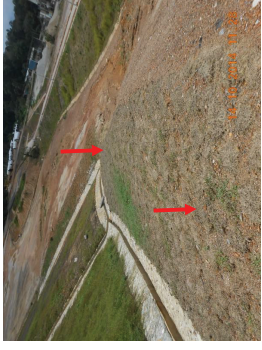
Plate 3a: Turfing has been dead is observed (Main Dam).
