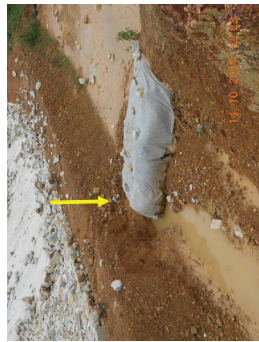
Plate 3a: Gap is observed at gabion wall (ST-2-16).
