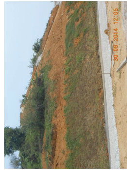
Plate 1f: Exposed slope is observed (d/stream spillway).
