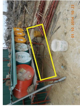
Plate 5b: Oil drums without tray are observed (saddle dam b).
