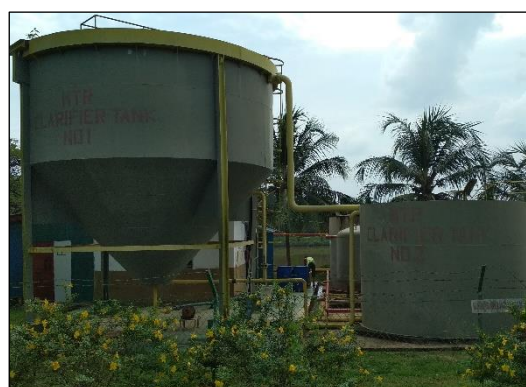
Plate 6.84: Samudera Estate water treatment plant
