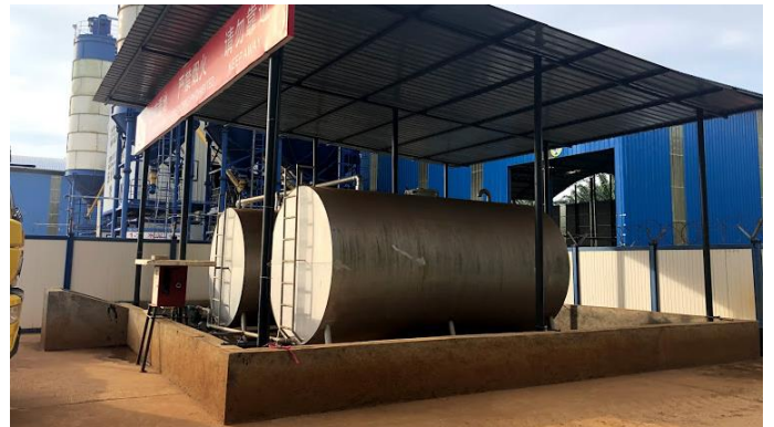
Skid tank stored in cement bund wall
